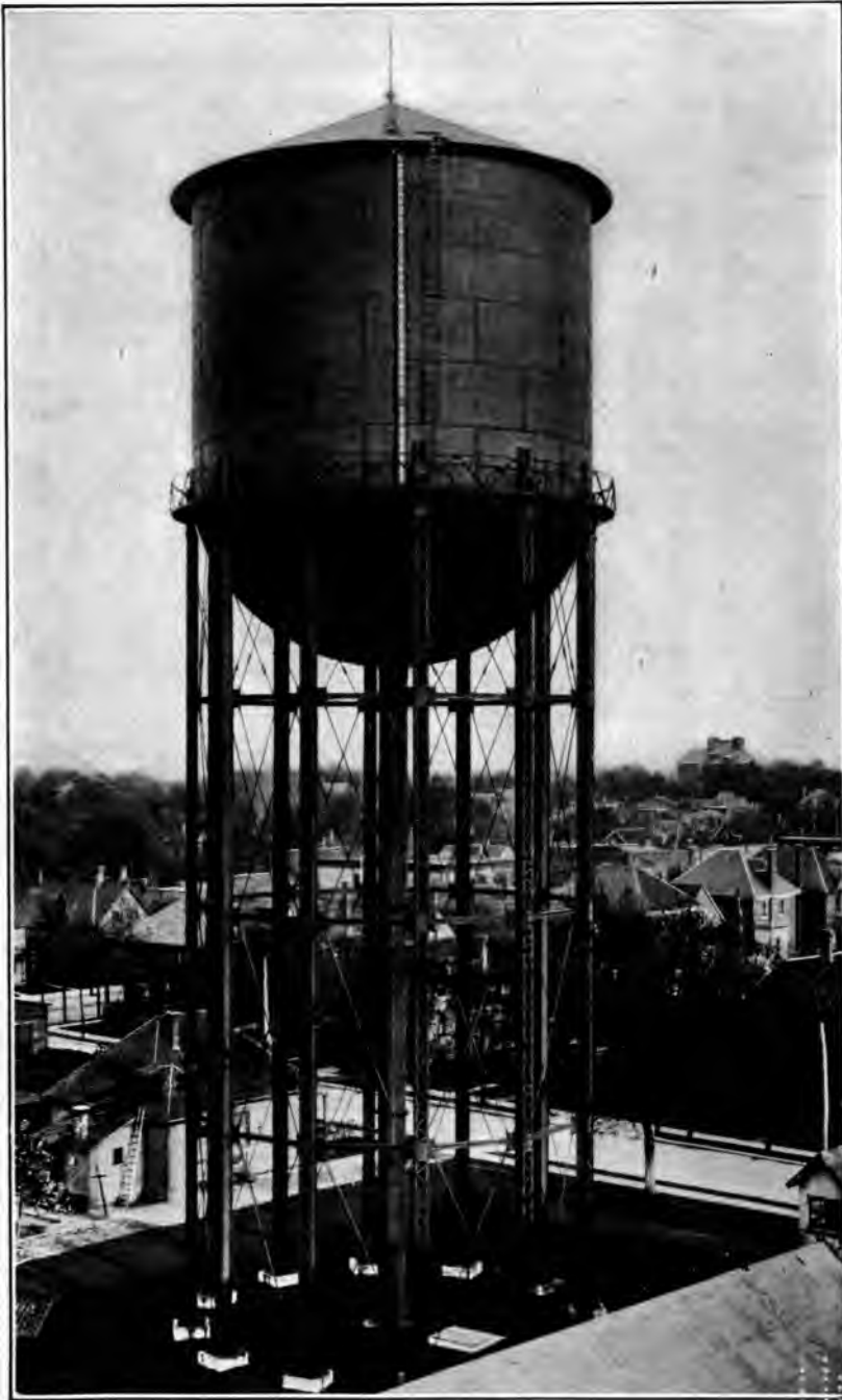
Steel Water Tank at St. Thomas, Ont. — Capacity 600,000 gallons. (Built by Pittsburgh-Des Moines Steel Co.)
